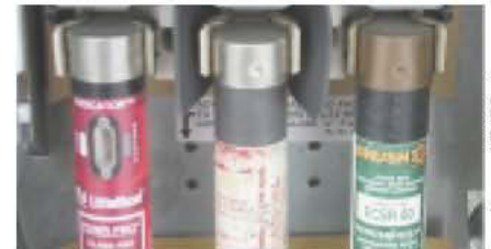
Visual image of a fuse panel.
