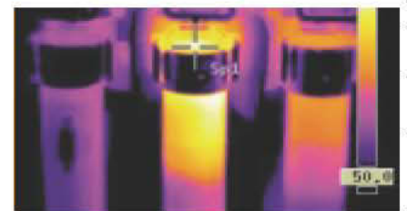
Thermal image revealing a hot fuse in the panel (yellow, orange, and red areas).
